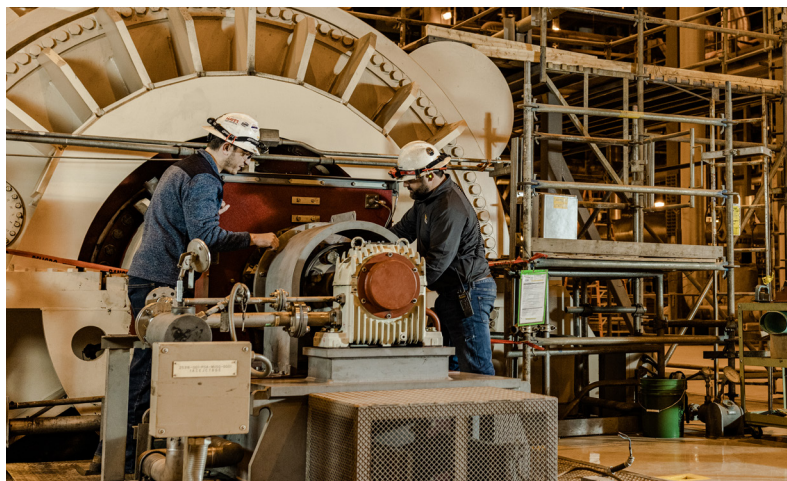
Technicians perform preventative maintenance on a generator at the Prairie State Energy Campus.
